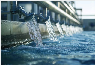
Centralised industrial water treatment and filtration system*
