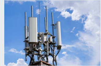
High-speed broadband and telecommunications infrastructure*
